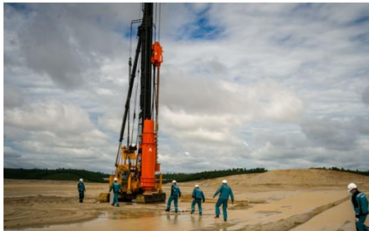
Ground was broken on August 18 in Russia's Far East on a massive $11 billion project that will result in one of the world's largest poly-
