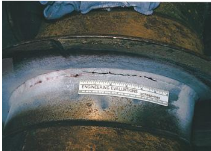
Figure 1.5 Shows the crack development at the end of shaft or weld section due to the stress and deflection, reference [9]
