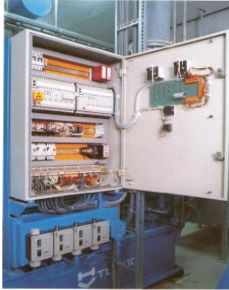
Fig 2.6: Local control panel for operating the HV turbo air compressor
