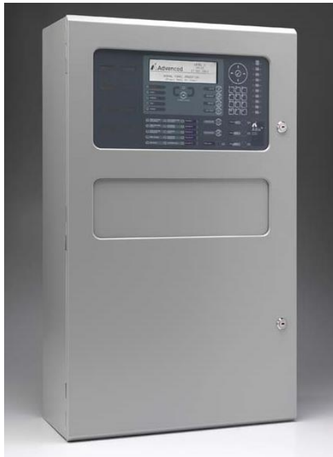
Fig. 3.29 Axis 8 Loop Fire Panel [38]
