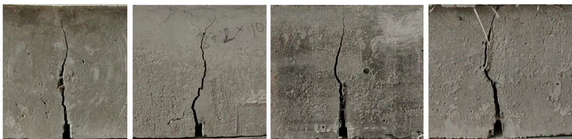
Figure 4. Concrete cracks after the test.
