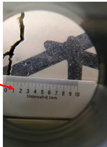
b) Zoom view of tightened sample till \leq 0,4 mm width crack
