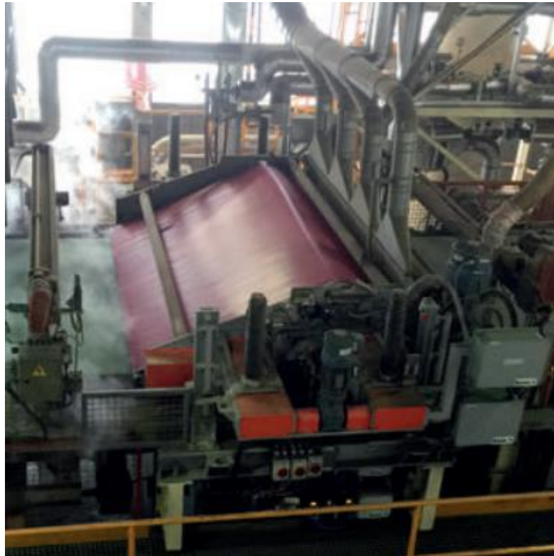
Fig. 25 Real picture of the steam injection equipment
