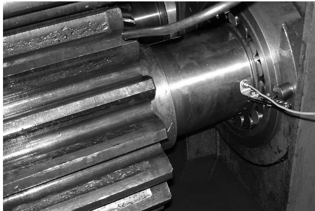
Fig. 2. The view of driving gear z_3 teeth damages and the II rotor shaft displacement and vibration displacement measurement with contactless sensor
