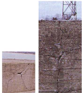
Fig. 2. Cracks of the concrete surface at the object
