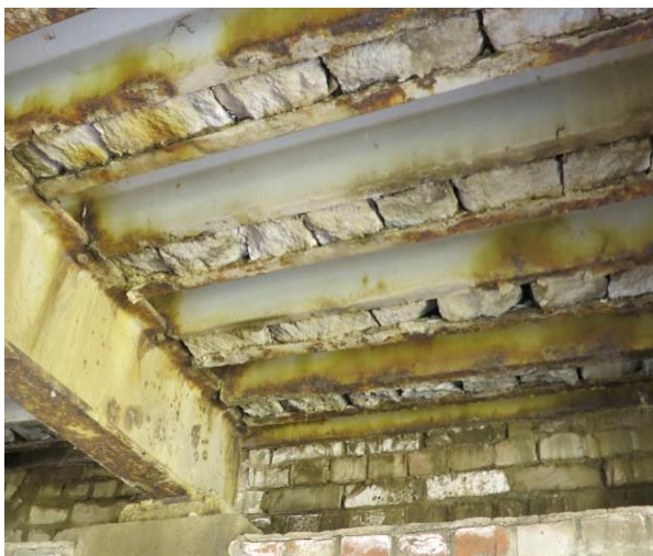
Fig.17 Bottom end stringers corrosion
