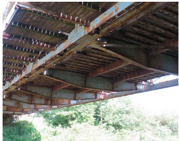
Fig 18 Lateral and cross beams corrosion
