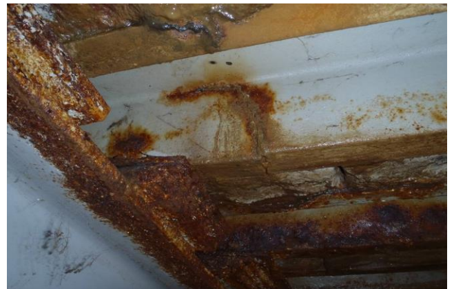
Fig.23 Stringer crack due to the corrosion
