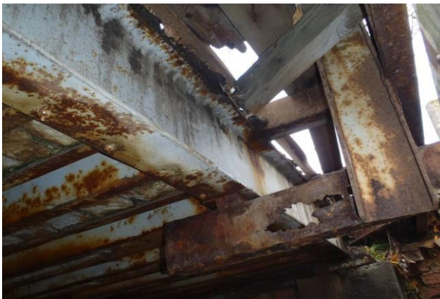
Fig.22 Bottom end corrosion damage
