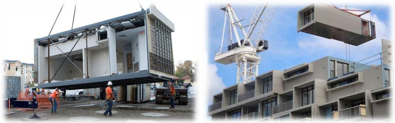
Figure 13 It Show the Erection of Building Part by part by using Crane “Source: Containex.co.uk, Modular Building”
