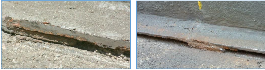
Fig. 2.3.1. Lap joint condition in a real storage tank floor during service and operation period
