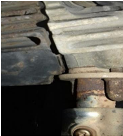
Figure 3 Crack due to lack of fusion and visible result of corrosion
