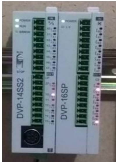
Fig.4.2. DVP-14SS2 PLC and DVP-16SP I/O extension unit
