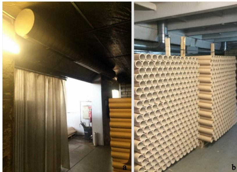
Fig.2.8. Drying station with a) closed entrance and b) heated air drying system
