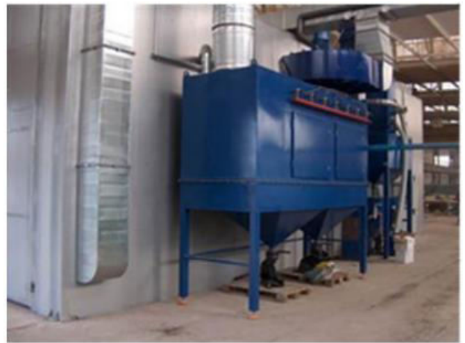
Fig. 6.4 Ventilation and dedusting equipment
