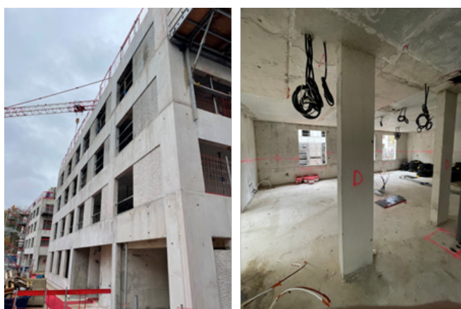
Fig. 1, Construction site I3F (France, 2022). All concrete on the photo is based on GGBS activated by Na 2 CO 3
