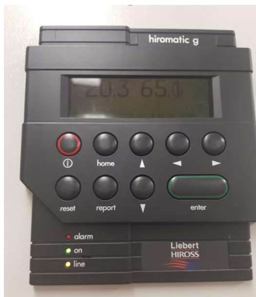
Fig. 12. Air-conditioning panel showing air temperature and humidity
