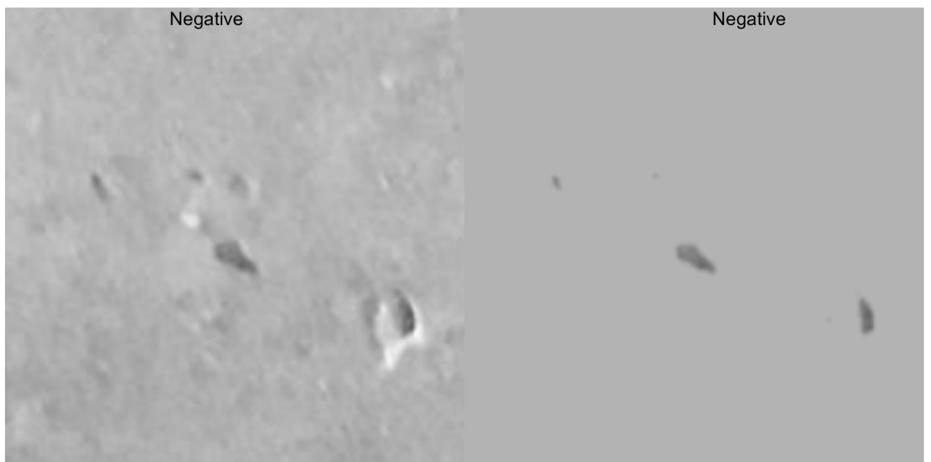
24 fig. Segmentation of lightly damaged concrete walls
