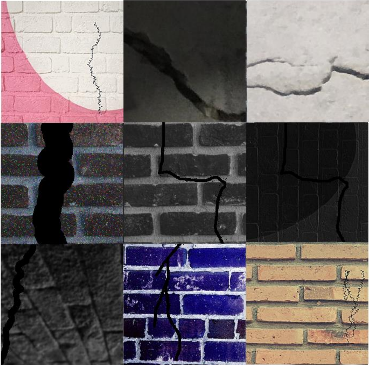
6 fig. Examples of crack images in our database
