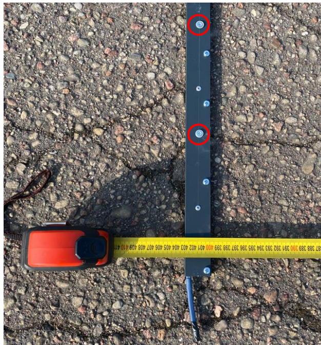
Fig. 49. Fixation of piezoelectric sensors with anchoring screws (marked red) on the road pavement
