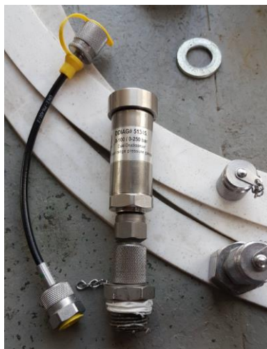
Fig. 5.3 Electronic monometer used for pressure test
