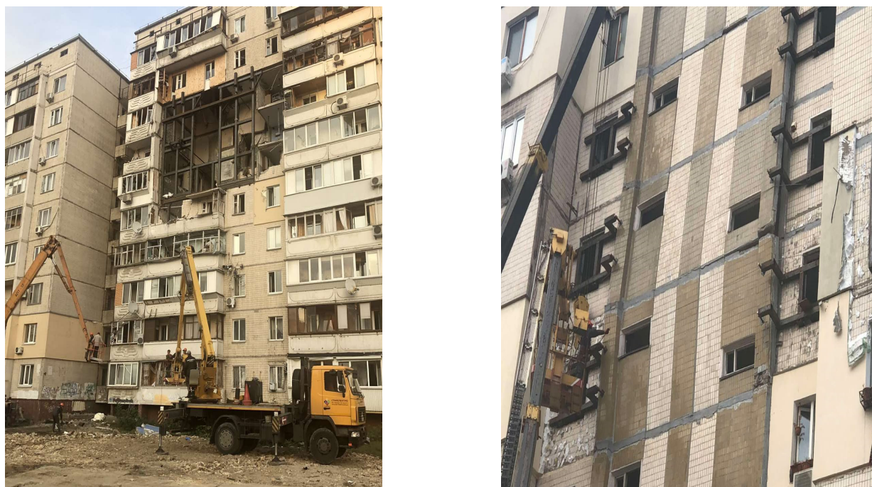
Figure 10. Urgent temporary stabilization of a large-panel building damaged as a result of a gas explosion (Kyiv city, S. Krushelnytska Street, June–October 2020).
