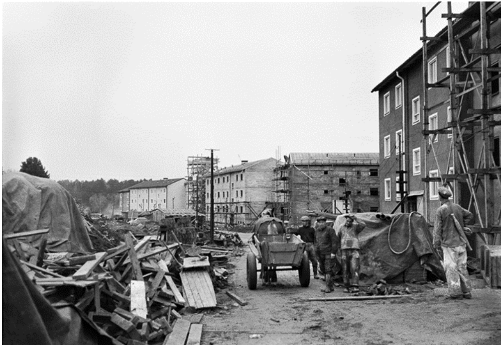
Fig. 11. Vällingby, construction of residential area (photo by Herman Ronninger. Svenska Dagbladet CC: License: BY)
