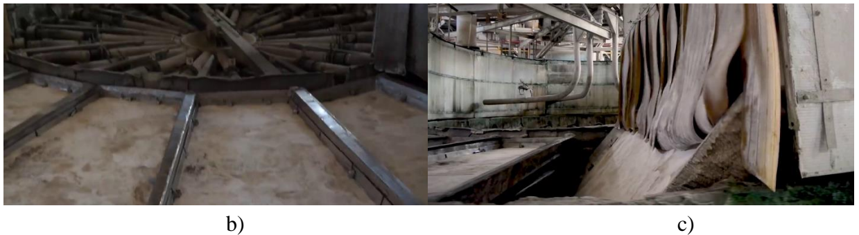
Fig. 5. Cake tilt-pan vacuum filter: (a) principal scheme of phosphoric acid pulp filtration [15]; (b) phosphogypsum filtration/drying stage; (c) phosphogypsum discharging stage
