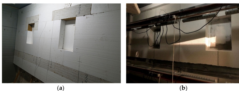
Figure 1. (a) EPS thermal insulation with mineral wool fire barriers; (b) test rig with 4 types of plastering during the test.
